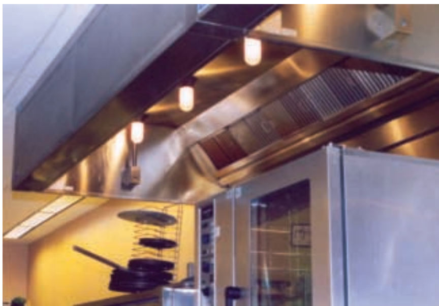
Optic sensors monitor smoke and vapors and adjust fan speed automatically.
