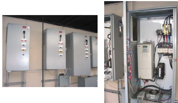
Figure 10. Variable Frequency Drives (VFDs)
