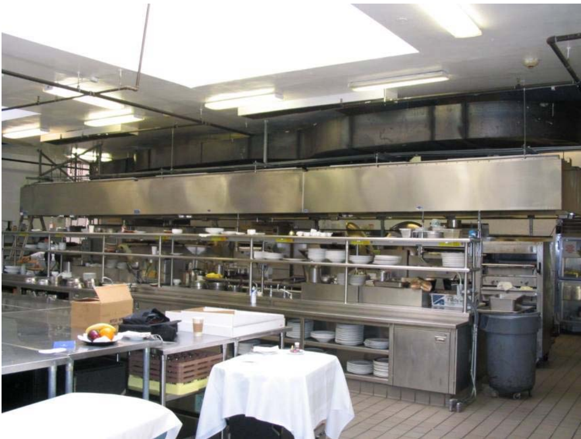
Figure 2. The Mark Hopkins Hotel Kitchen
