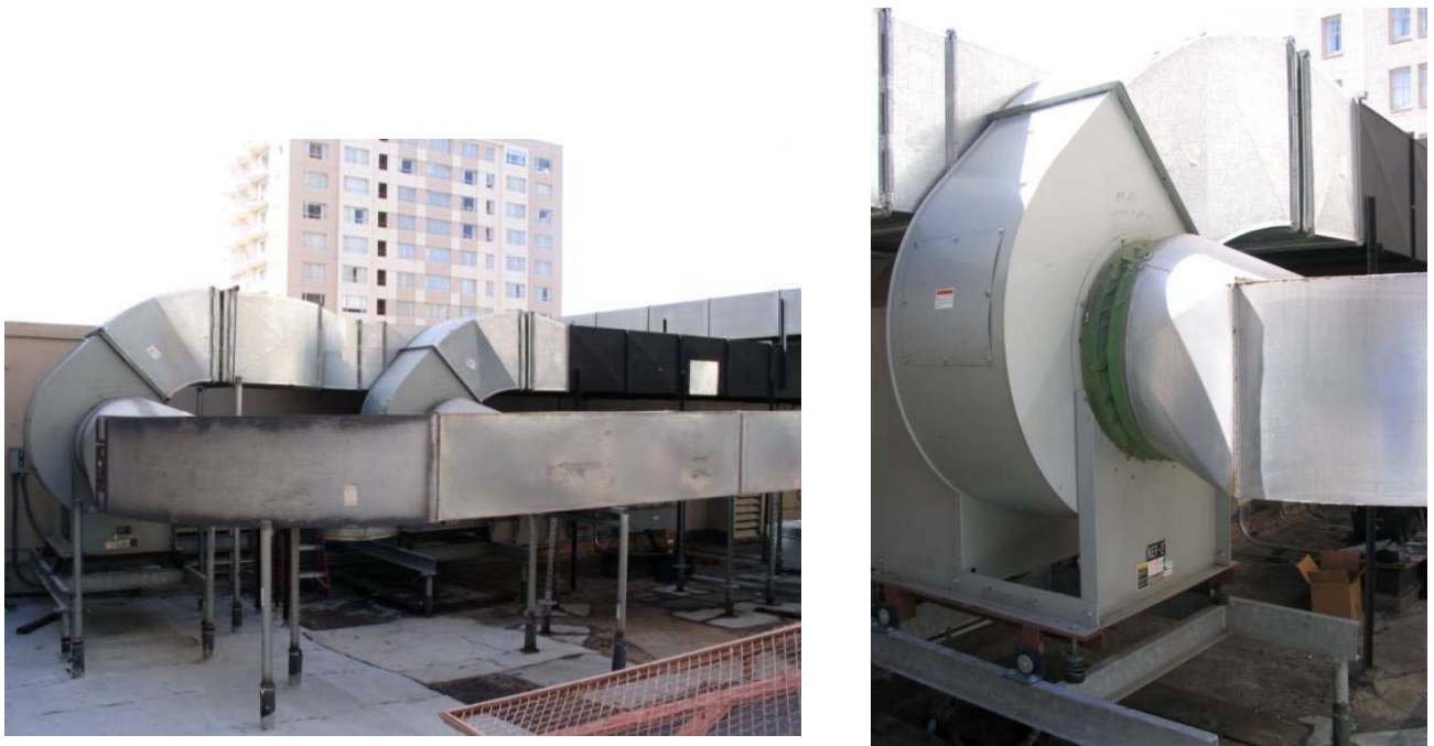
Figure 5. The Two Greenheck Exhaust Fans
