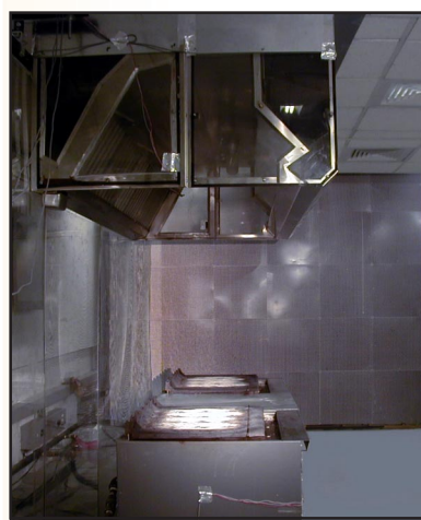
Two 3-ft. charbroilers under an 8-ft. wall-mounted short-circuit canopy hood.
