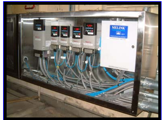
Figure 6: The VFDs and I/O processors had to be installed in a cramped attic mechanical room. This made installation a challenge.
