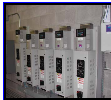
Figure 11: VFDs used to control the four of the exhaust fans and the make-up air handler fan.
