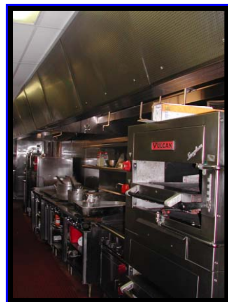
Figure 10: One of the cooking lines at Hyatt Regency Sacramento.
