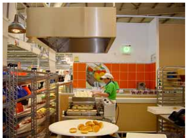
Doughnut frying extract now Intelli-Hood controlled
